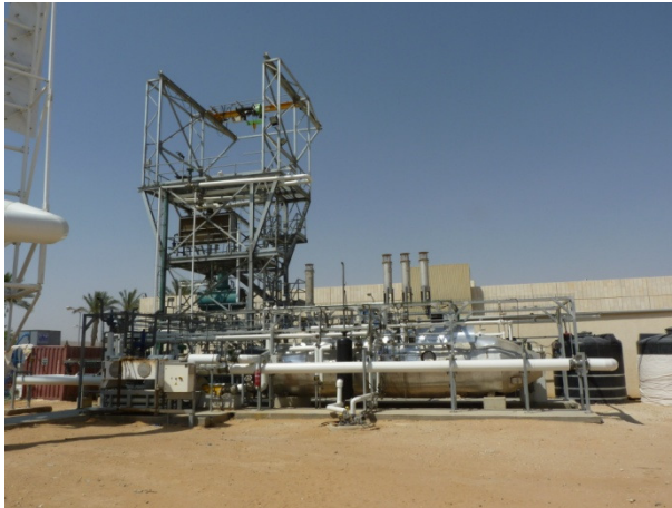
Fig. 4: Heat exchange system and maintenance tower
